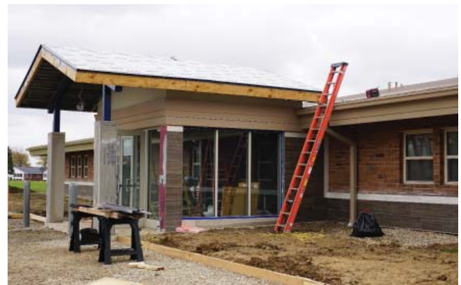
A new entrance will greet visitors at Mercer DD's Mud Pike facility west of Celina.
